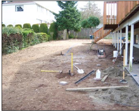
Before: This lawn was a problem to keep healthy, and the homeowner a nice yard.
